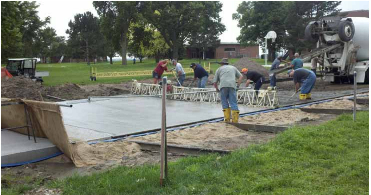
One of 10 concrete pours for the new road at the Youth Rehabilitation and Treatment Center in Kearney.
